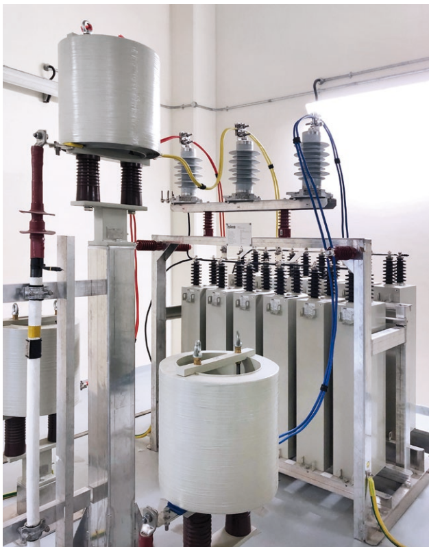
11kV 5MVAR project
